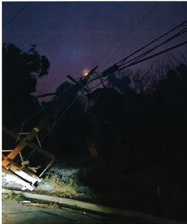
28 LADWP Pole No. 126531M During the Palisades Fire
