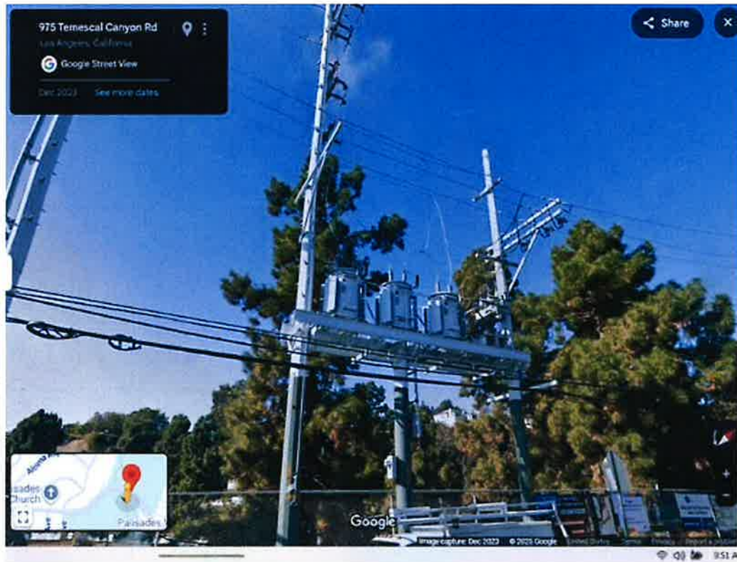
Pole Top Distribution Station 195
